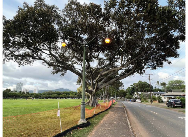
Work on the Kapi'olani Park pathway will begin at Monsarrat Avenue & will progress towards Diamond Head
